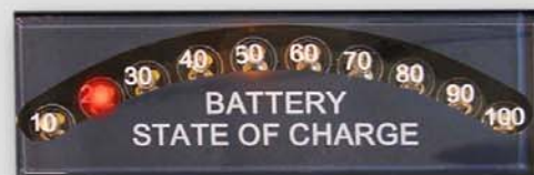
Batteries have only a 20% charge
