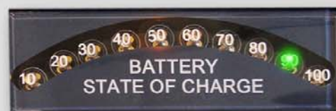
Batteries have a 90% charge
