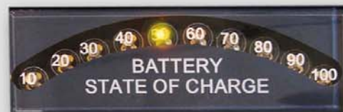
Batteries have a 50% charge
