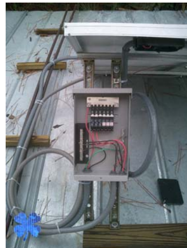
Installation photo by Maverick Solar
