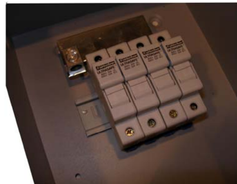
Fuse holders in enclosure
