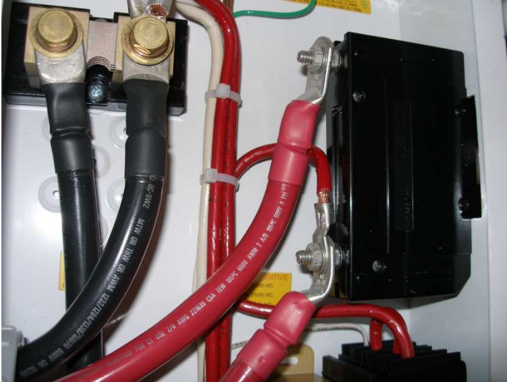
Battery Positive connections and shunt wiring
