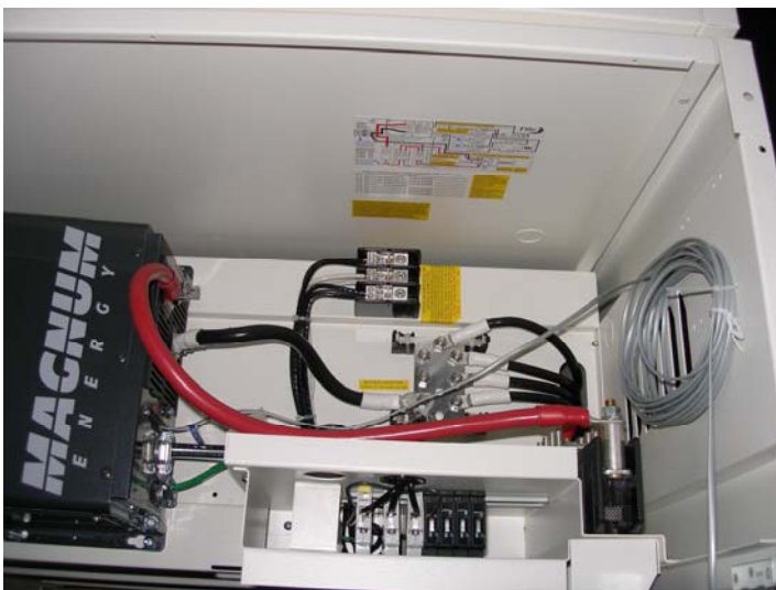
Photo of AC terminal block compartment
